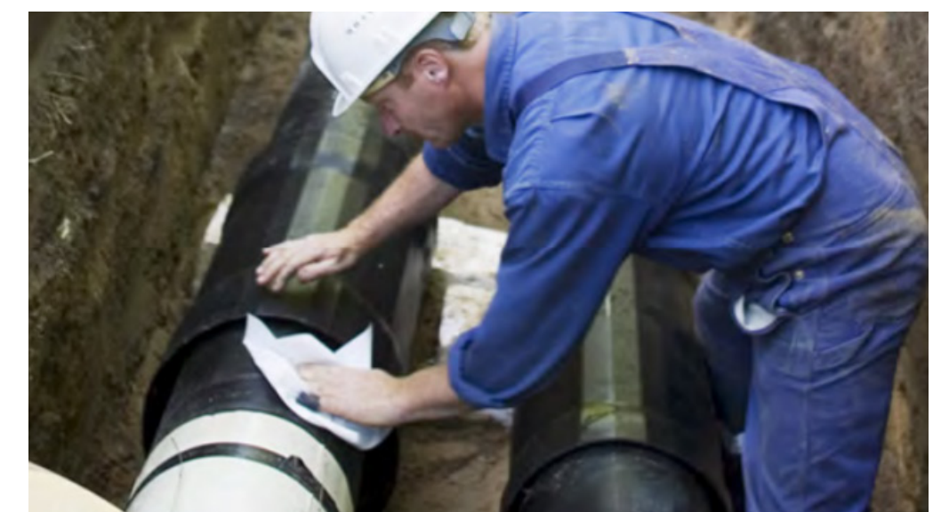
Image: Underground Insulated Pipes This system is used to transport hot or cool water to and from the district heating plant.
