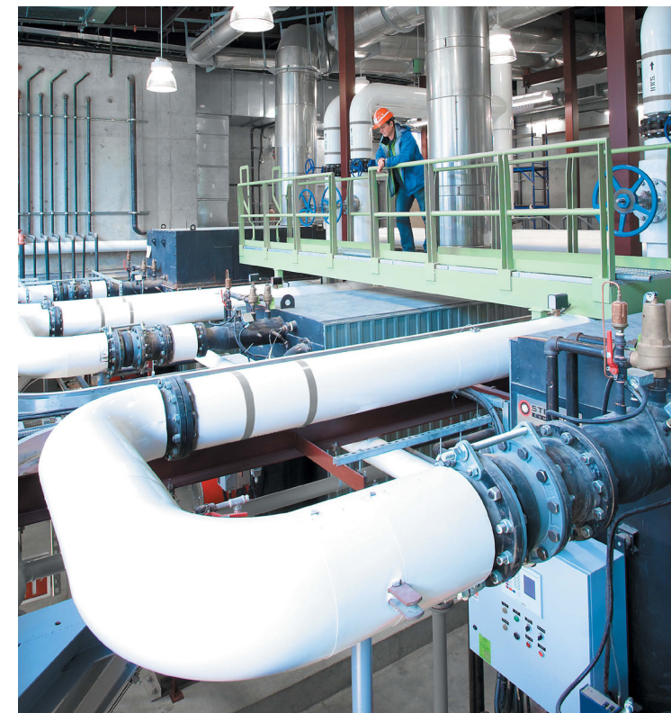
Blatchford District Energy Sharing System Edmonton, AB, Canada
