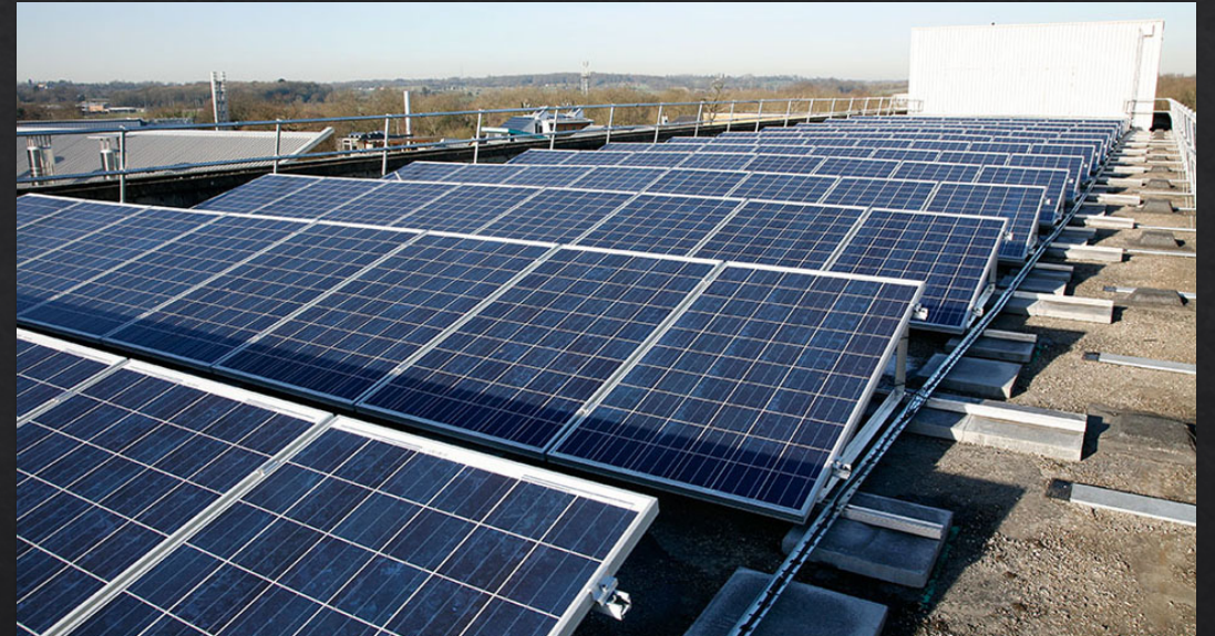
Solar Roofs – 12.5% of site coverage
